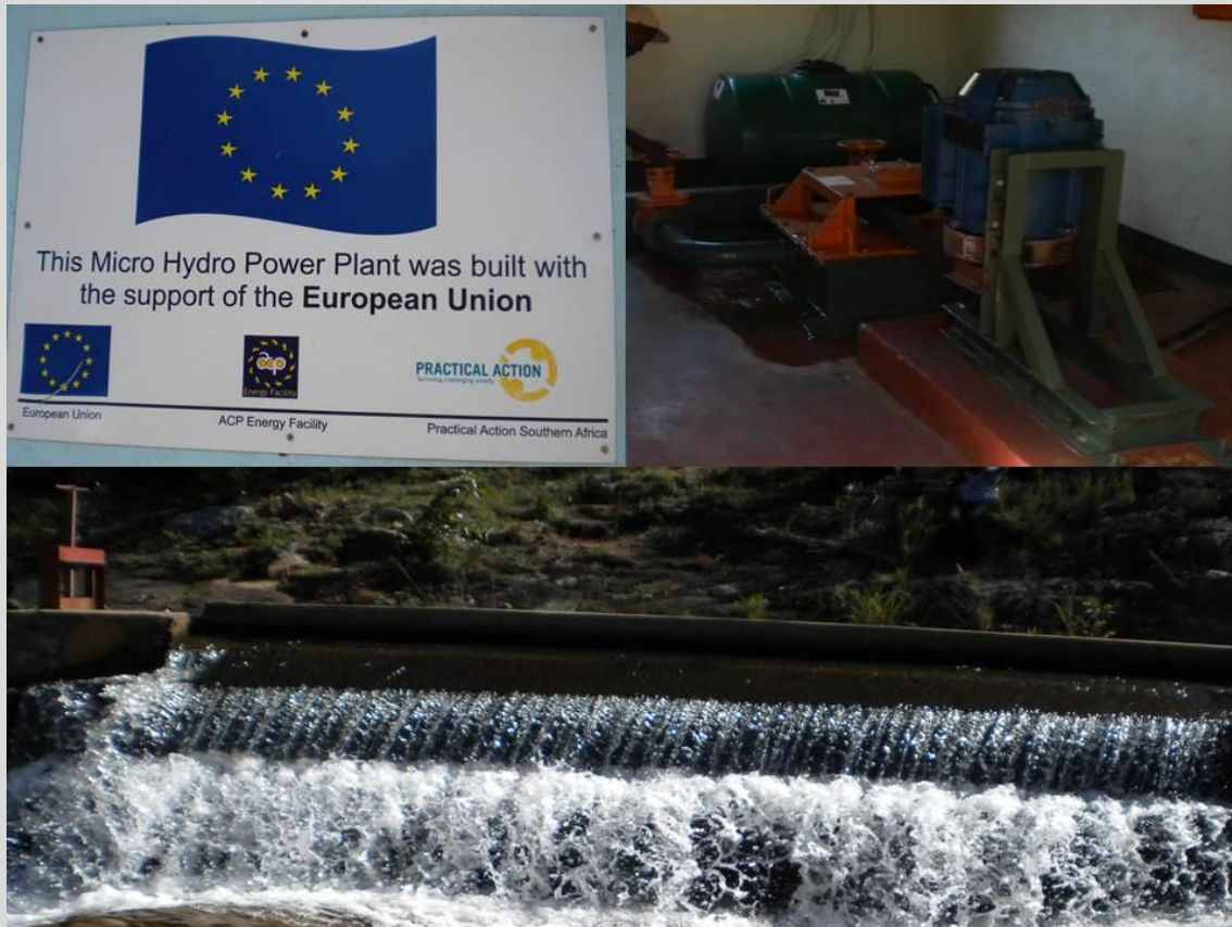
Figure 4: Chipendeke mini-hydro power plant
